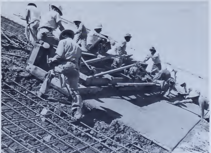
Figure 145.—Job-built slip form being used on sloping apron of left abutment of Nimbus Dam, Central Valley project, California. Reinforcement is systematically tied and supported on concrete blocks. Notice pattern formed by using V-grooves at construction joint of abutment in background. AR-1523-CV.
